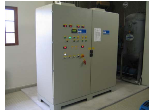
Daon, France 1.6 MGD
