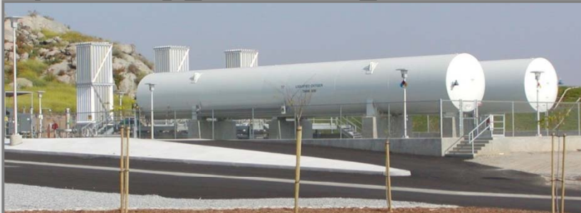
Liquid Oxygen Storage & Ambient Vaporizers
