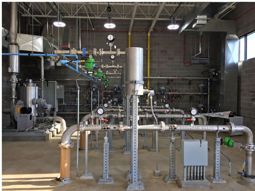
A set of sidestream injection systems enables WaterOne to adapt to a 12:1 turndown ratio.
