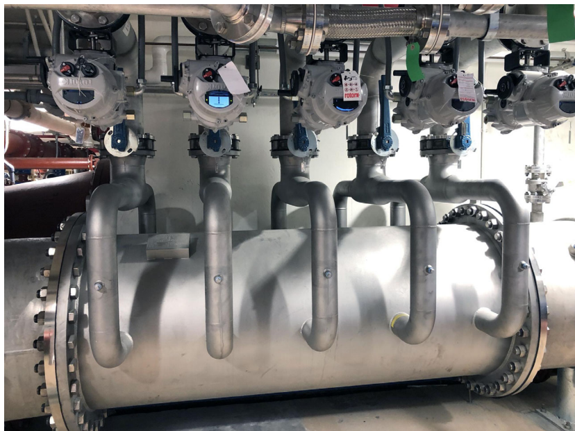
Maintenance on the Orlando Utilities Commission's Pipeline Flash Reactor is quick and easy compared to draining fine bubble diffusers and working in enclosed spaces.
